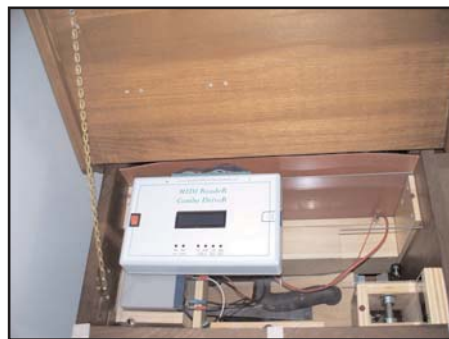
Figure 2. The new MIDI unit installed.
