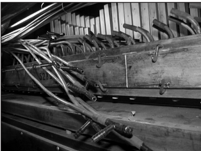
Figure 5. Another view of the Bruder valve chest showing some tees attached to the lead tubing.
